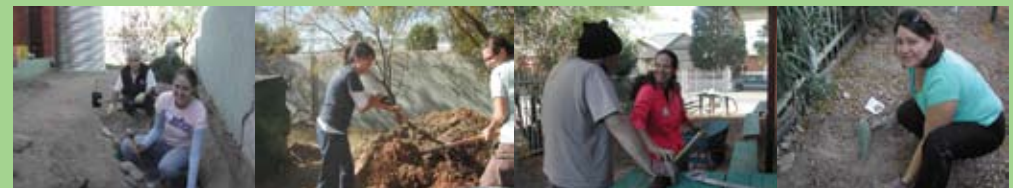
Installation of a water harvesting system for our garden, funded by the Blue Water Project Grant. Thanks to all our volunteers and staff for a successful workday at BorderLinks!
